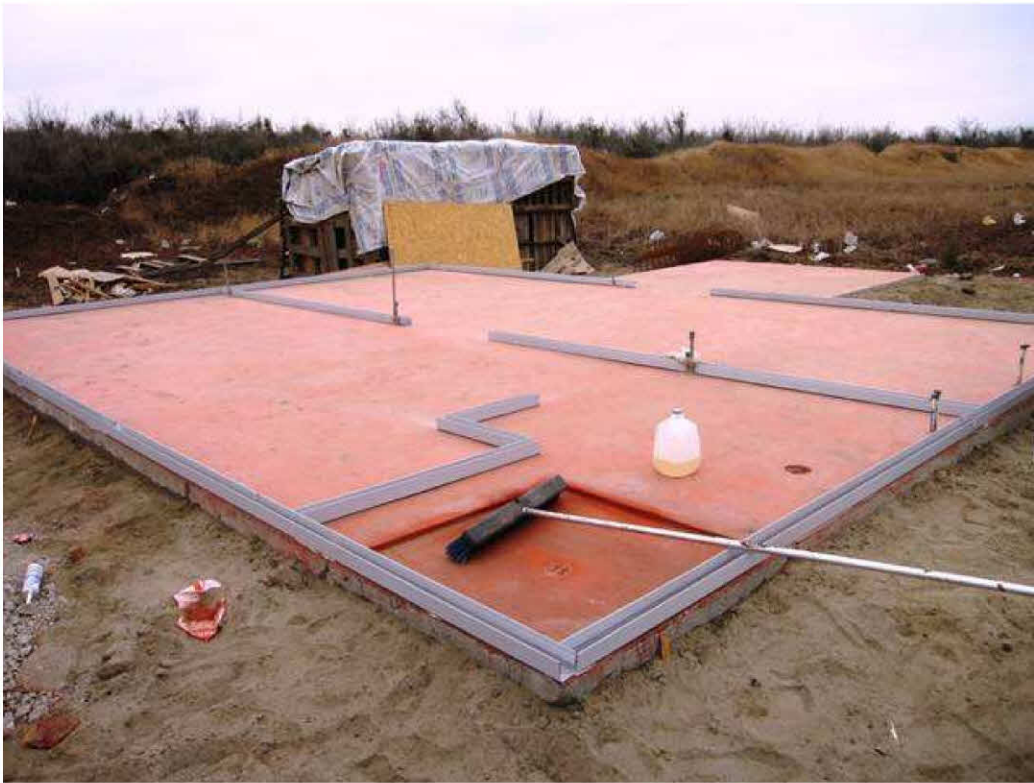
The concrete pad with new U channel layout. Note the family's current house in the background.
